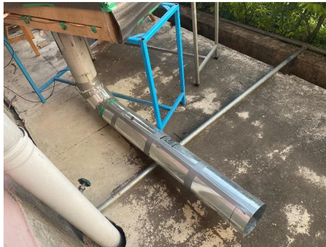
Figure 3-6: Dryer's inlet extension
