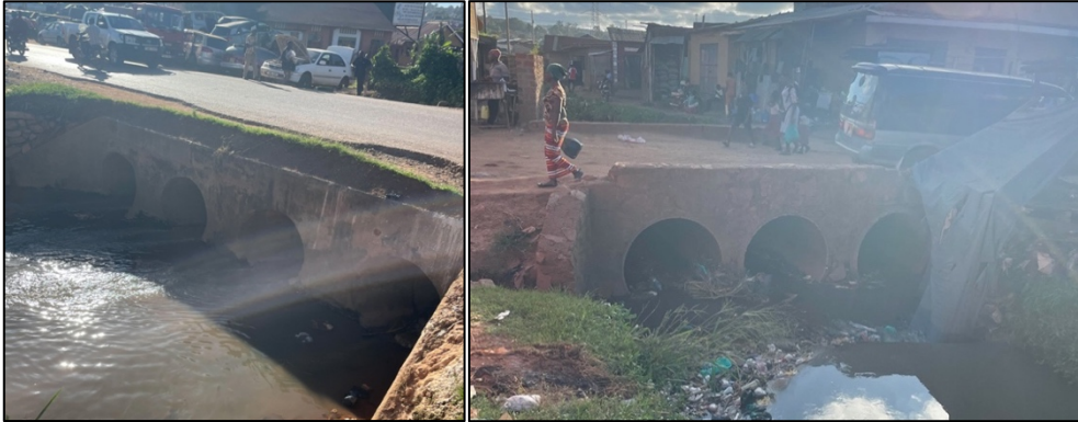
Figure 25 Culvert crossing at Alice Kaggwa Road (to the left) and Kamwokya Kisalosalalo Road (to the right).
