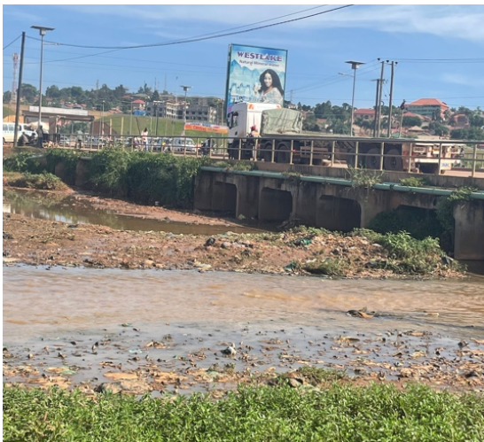
Figure 3 Silt- and solid waste in Lubigi primary channel
