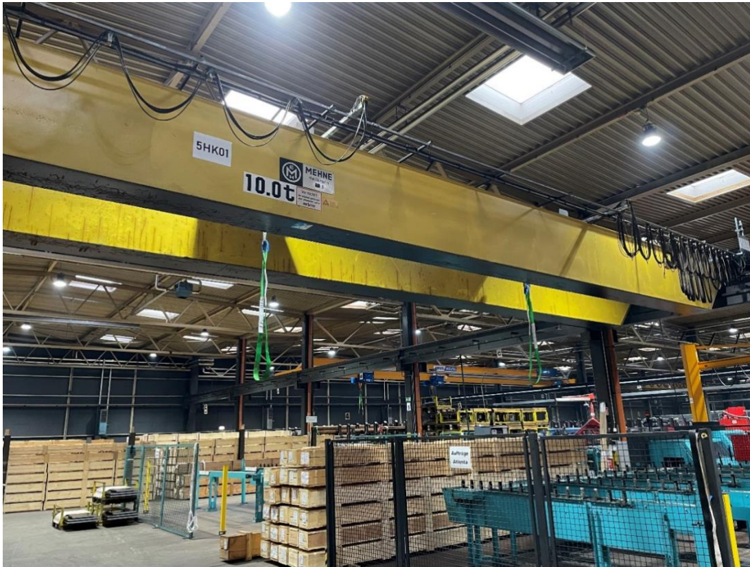
Figure 25: Overhead crane in the warehouse of Heine + Beisswenger.
