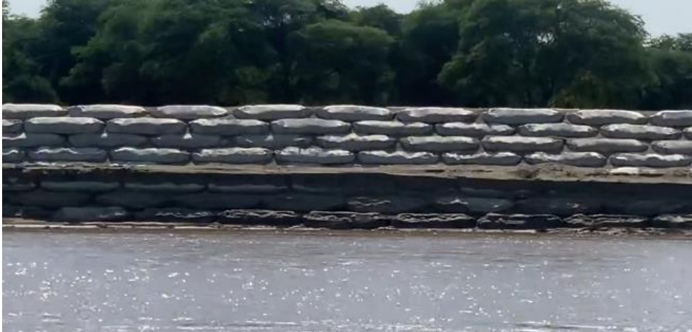
Figure 29- Erosion close to Drain 13.08
