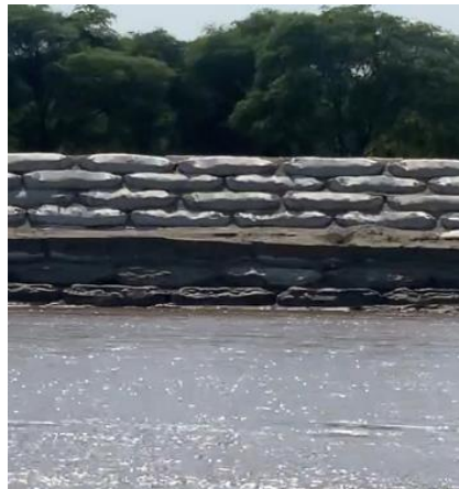
Figure 34- Erosion close to Drain 13.08
