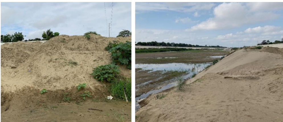
Figure 25- Sediments at Los Ejidos dam. 25a- View from bottom. 25b- View from top
