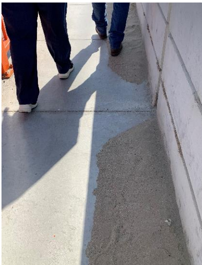
Figure 25- Eolian Sediment on Bridge
