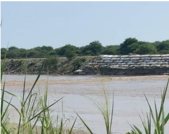
Figure 33- Drain 13.08 crossing through Piura River
