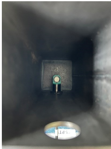
Figure 5.7 Ultrasonic sensor mounted in steel profile.
