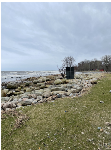
Figure 1.3: Erosion along the top of the rock revetment at Kivik WWTP
