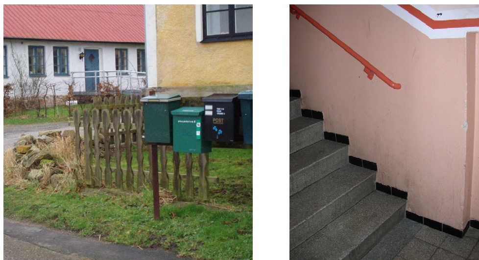
Figure 6. Two of the core environmental barriers identified. Letterboxes can only be reached via differences in level (left), and handrails are too short (right).
