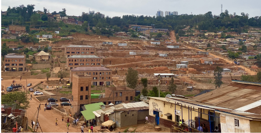
Figure 22: Removal of more informal settlements and preparing the foundations of Block E-W.
