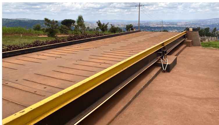
Figure 13: The recently installed weighing bridge.
