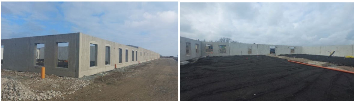
Figure 6 The poultry building under construction in Borby Sweden which is used as an example for Conventional construction in concrete and steel. Photograph taken by author:
