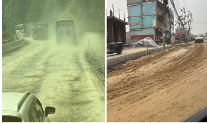
Figure 5.10: The left photograph shows the damaged road between Kathmandu and Pokhara, and the right shows how the road between Kathmandu and Banepa deteriorates after rainfall.
