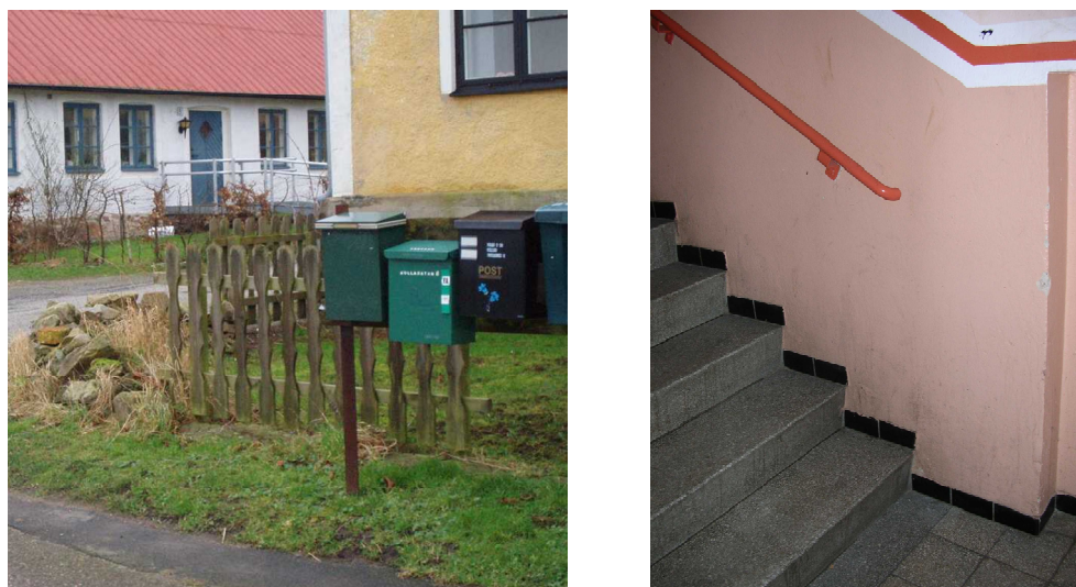
Figure 6. Two of the core environmental barriers identified. Letterboxes can only be reached via differences in level (left), and handrails are too short (right).
