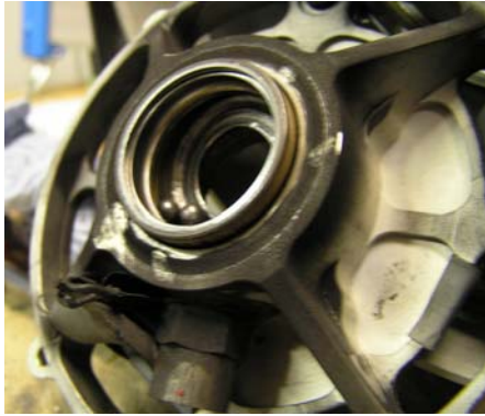
figure 36 , the bearing sleeve covered with dust.
