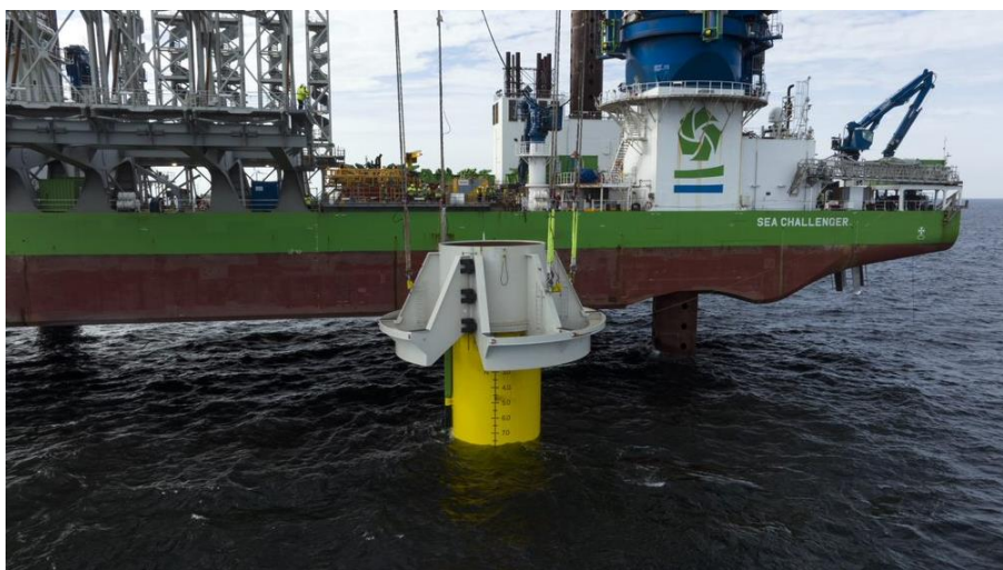
Figure 4: Installation of a steel collar, photo by DEME Group (RWE Renewables n.d.).
