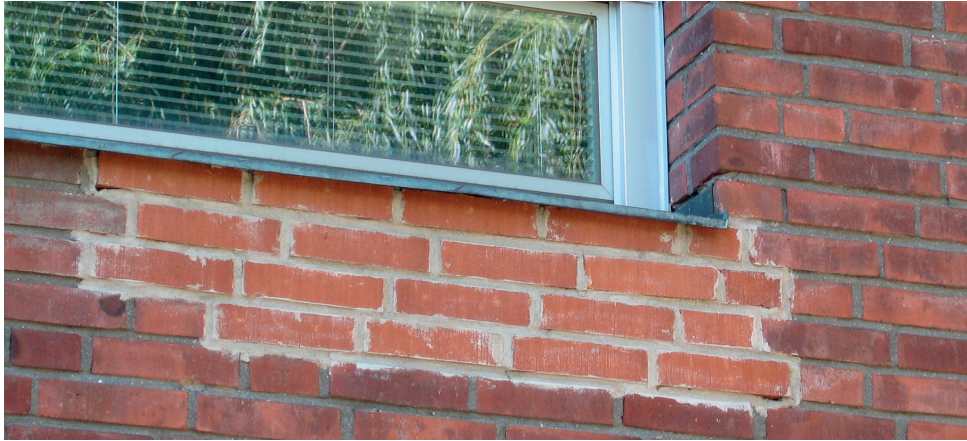
Figure 2. An example of adverse effects of selecting unsuitable mortar and shoddy workmanship on repointing
