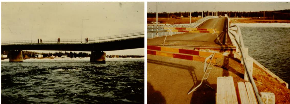
Figure 17. Failure of the bridge over Lainio River due to scour (from Dargahi, 1982)
