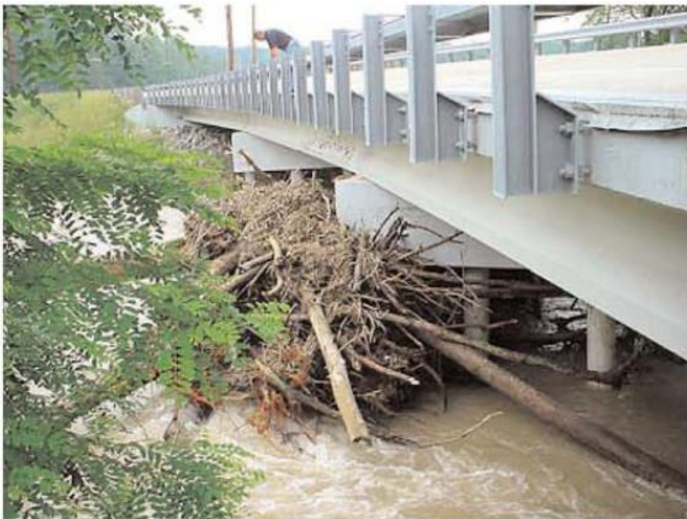
Figure 26. Example of debris accumulating at bridge piers (Lagasse et al., 2010)
