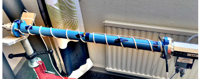
Fig. 1. Rigid coaxial line with directional coupler (to the right) used in the phase-reference distribution system at ESS. Sensors for surface measurements of the temperature and a heating cable wound around the outer copper tube have been mounted on the coaxial line. The complete phase-reference line and directional couplers are then insulated (see Fig. 7).
