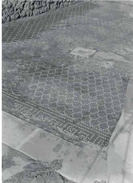
Fig. 72. Mortar-floor with an imbrication-pattern and a meander-threshold in the fauces of Cd Colombe a mosaico (VIII 2,34). View from atrium .
