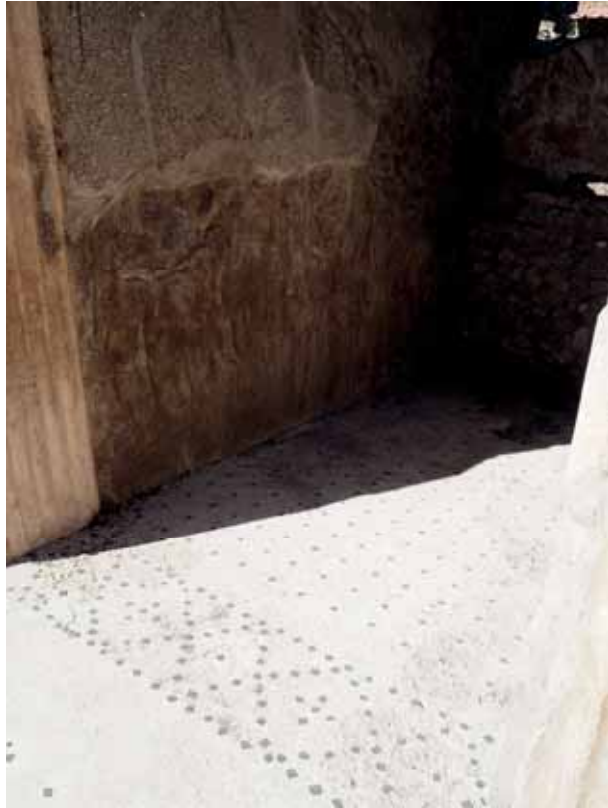
Fig. 68. White mortar-floor with rows of tesserae in the fauces of Cd Frutteto (I 9,5). View from atrium .
