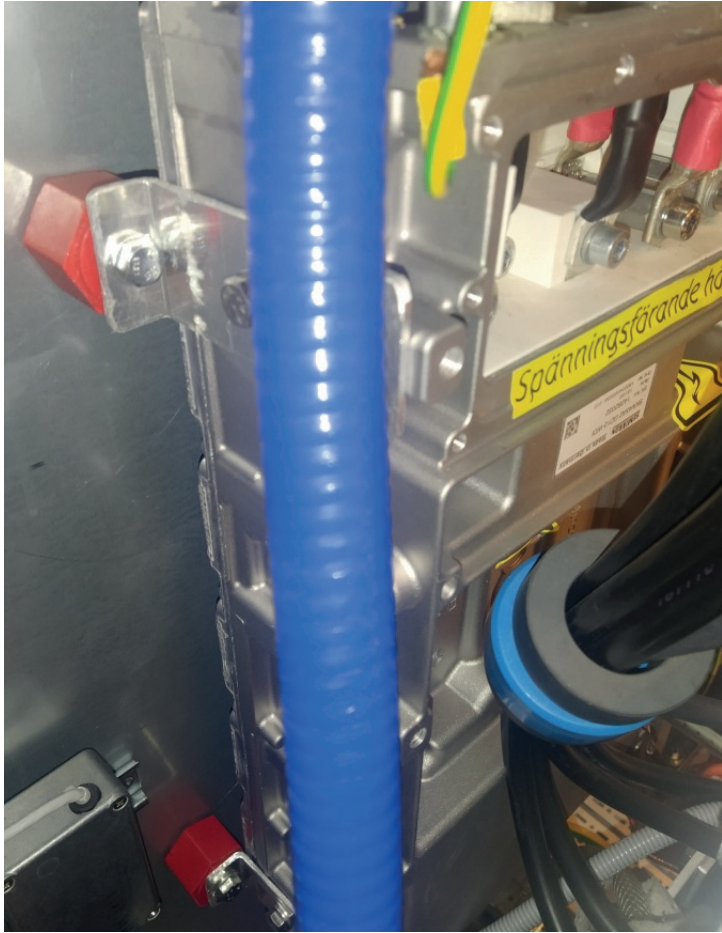
Figure A.4: The mounting of the traction converter in the electrical cabinet. The red mounting points are isolators. The blue hos in the foreground the coolant supply to the converter.
