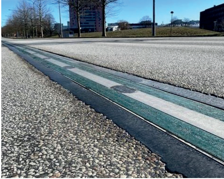
Figure 1.5: One of the test sites of road bound conductive ERS on public roads in Sweden. Photo: Elonroad
