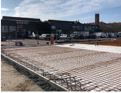
Figure 3.31. Construction of a new building in the northern part of the parking lot, 2019. Photograph by the author
