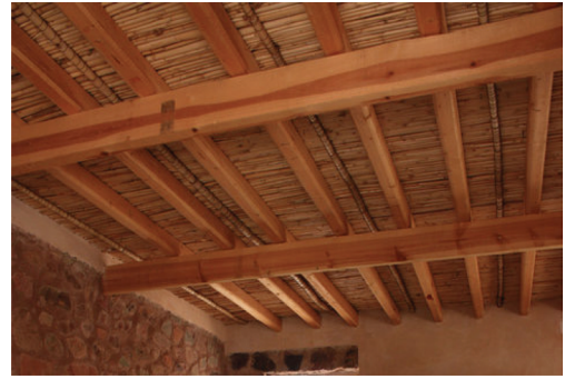
Figure 6. Roof structure developed based on roofing vernacular techniques in Saint Catherine. (Credits: Nashwa Ibrahim).
