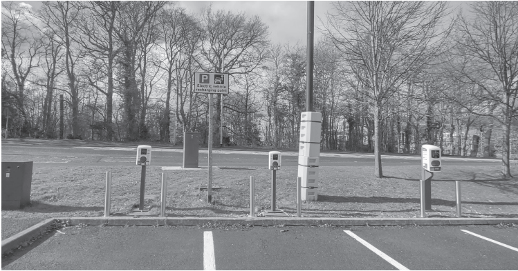
Figure 1: A trio of electrical vehicle fast chargers in a ‘park and ride’ on the outskirts of Durham. Their placement illustrates the difficulties that wheelchair users were complaining about with respect to the height of the charge points.
