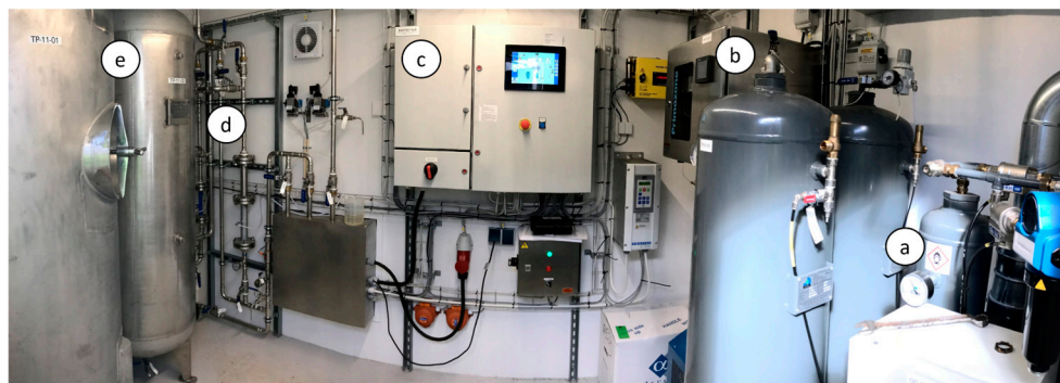
Figure 10. Photograph of the pilot-scale ozonation plant. Showing the oxygen generator units (a), ozone generator (b), control panel (c), ozone injection points (d) and reaction tanks (e).
