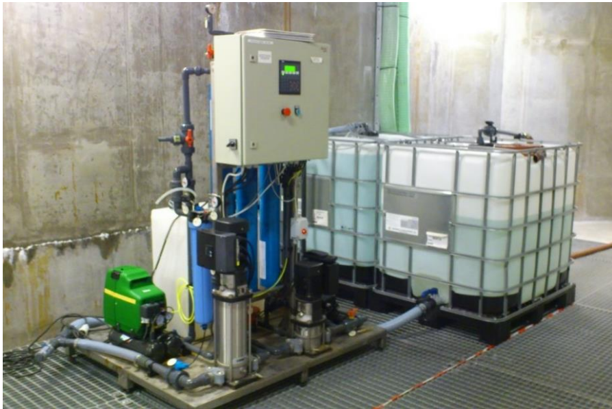
Figure 6 The spiral wound NF-pilot, placed in the basement of Ringsjö WTP.
