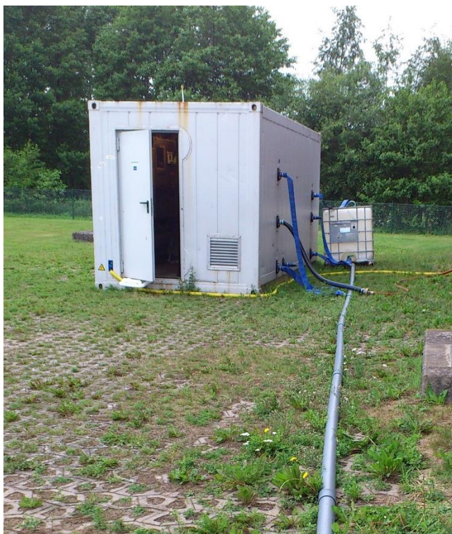
Figure 8 The NF-pilot 80 was located in this container, here placed at the pumping station of Ringsjö WTP.
