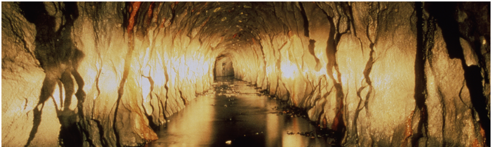
Figure 8: Photo of the Bolmen Tunnel from the inside taken during construction work (source: Sydvatten AB (2020))
