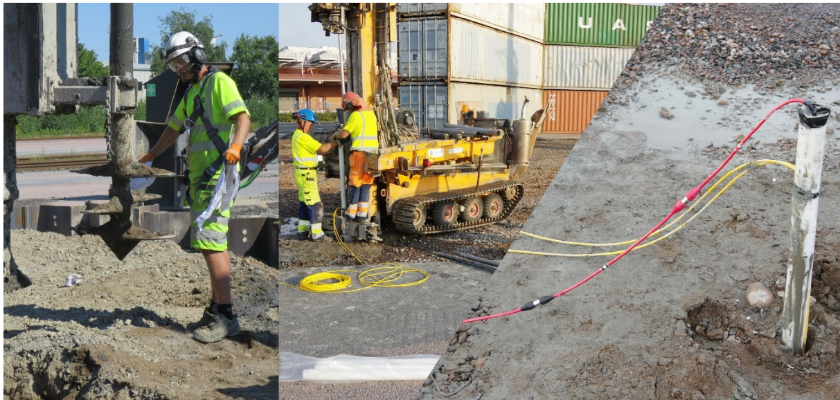
Figure 1 Documentation of the field installations and measurements: mixing tool with 80 cm diameter (left), installation of slotted PVC-pipe (middle) and installed ERT-cable (right).
