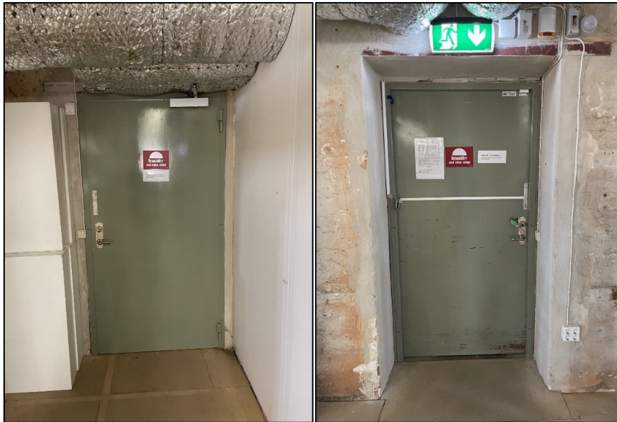
Figure 2. Design of the door. Inward opening side to the left, and outward opening side to the right.
