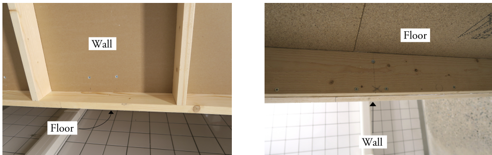
Figure 2.9: Photographs of a junction between the floor and a wall in the upper room. In the left photograph, the floor cannot be seen, but the arrow indicates its placement.
