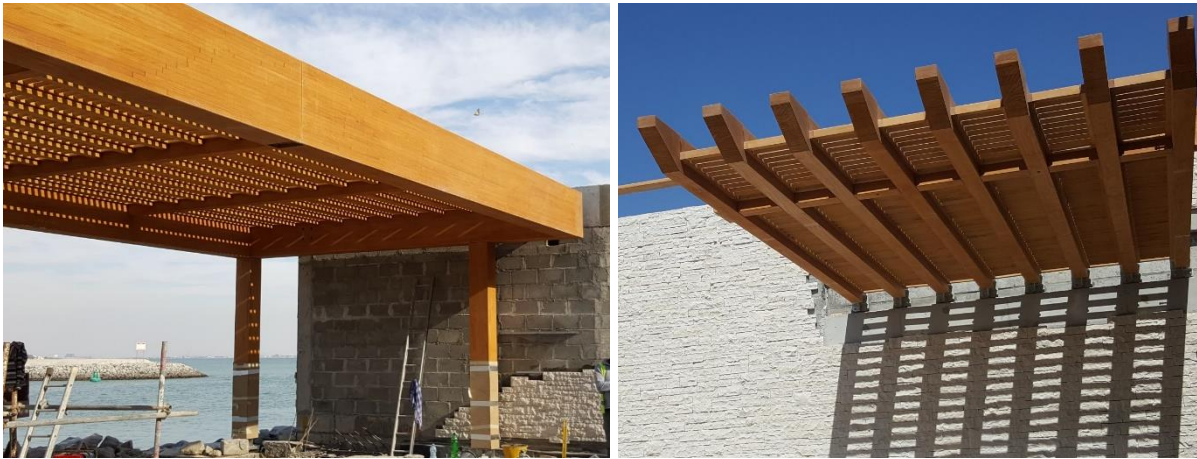
Figure 37. Examples of use in outdoor structures. Left: Portal frames with post/beam moment resistant connections. Right: Rafters with moment-resistant connections fixed on a wall.
