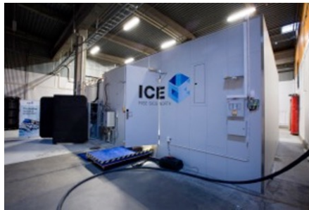
Figure 5.1 Small DC pod at RISE SICS North in Luleå, Sweden.
