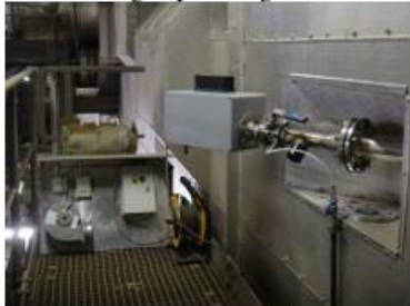
e. IACM receiver, cross-stack over a corner
