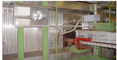
f. The receiver mounted on the full-scale CHP boiler during long-term measurements.
