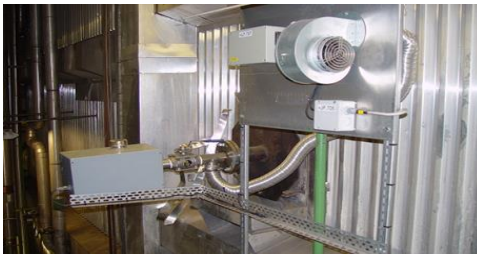
e. The transmitter mounted on the full-scale CHP boiler during long-term measurements.
