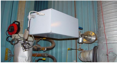
c. The receiver mounted on the research CFB boiler.
