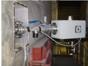
f. IACM transmitter, cross-stack over a corner
