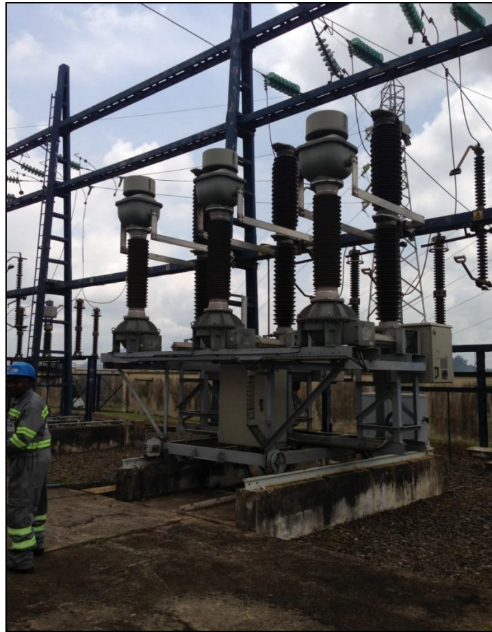
A modern African electricity substation.
