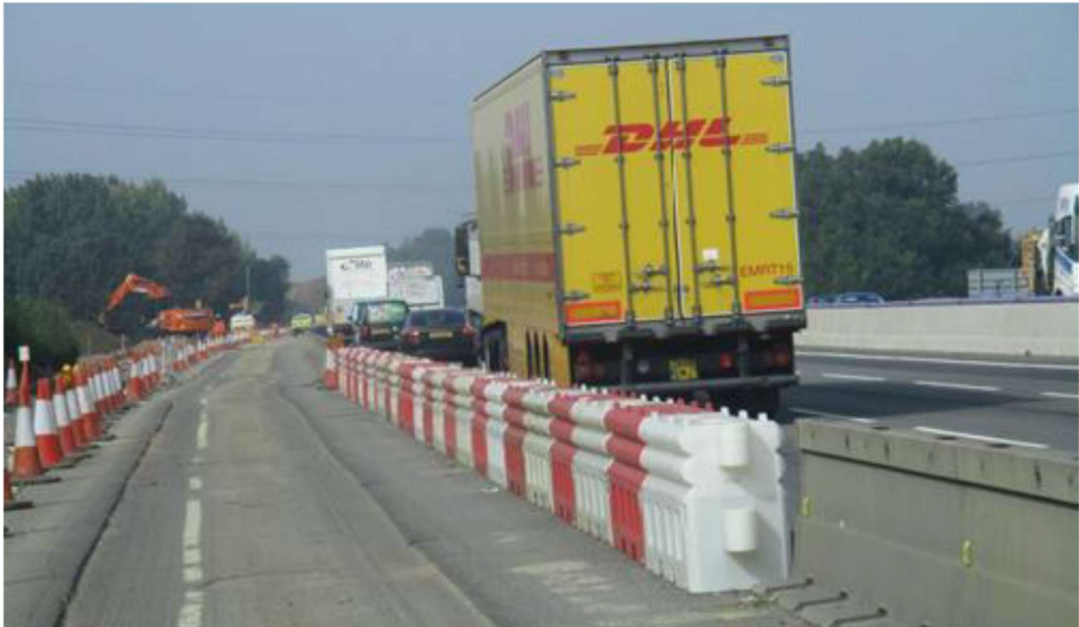
Figure 22. Water filled barriers filling the gap in the zone guard (Highway Safety Hub, 2018).
