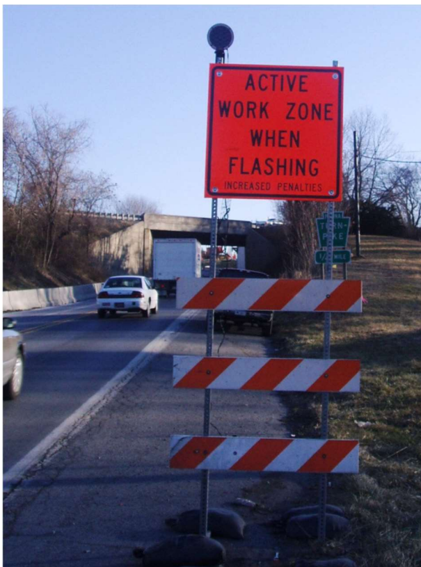
Figure 10. Work zone sign complemented with flashing light when road workers present at the site (Sesny, Lentz and Rensel, 2007).
