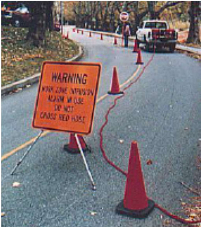
Figure 28. Pneumatic tube incursion alarm (Wang et al., 2013).
