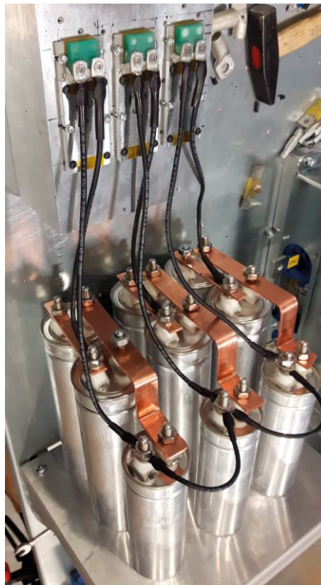
Figure 9.5: Overview of line filter capacitor branches. The capacitors in the damped branch of the filter are connected to custom-made damping resistors. Power dissipation is aided by the heatsink.
