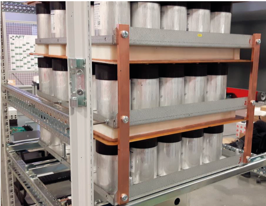
Figure 9.9: Overview of main capacitor bank.
