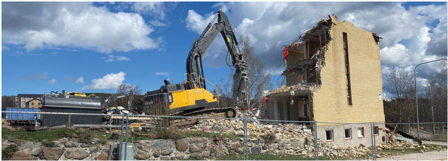
Figure 17. Houses prepared for demolition, sensed as to close to the mining pit and vibrations from explosions. (O7)
