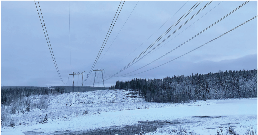
Figure 25. A photo taken on a walk through Jokkmokk (Q15), taking in the loud buzzing below the energy gridlines. (O15)
