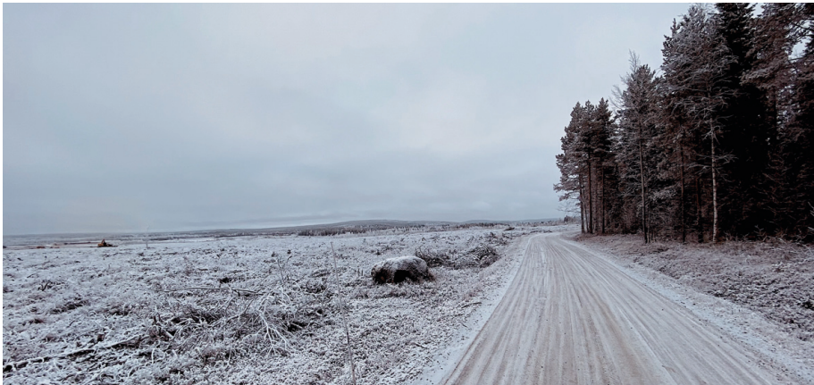
Figure 16. H2GS steel site to the left, after deforestation. Machines such as the one on the far left side even the ground.
