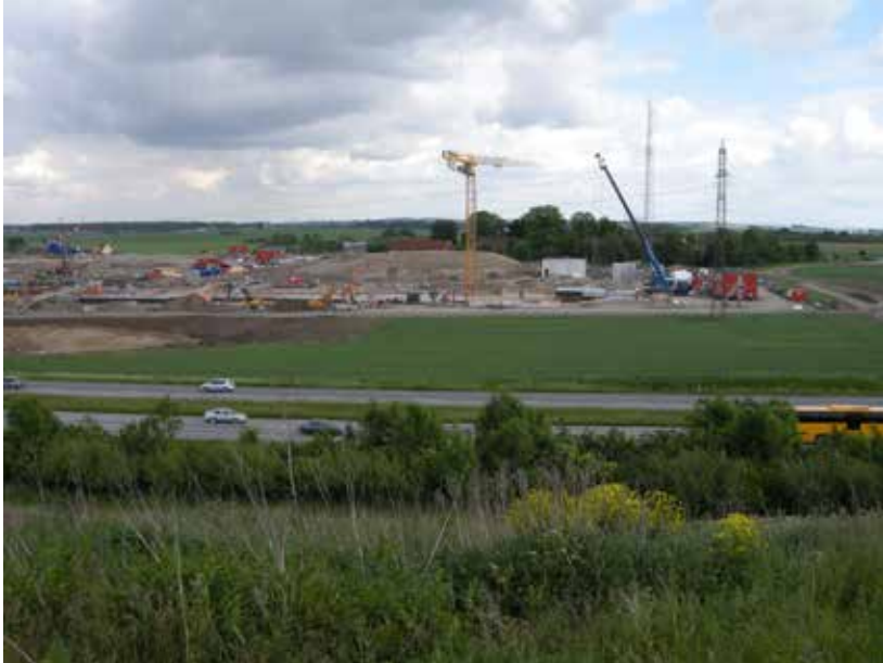
Figure 20. The view of the building site of MAX IV from Norra Fälåden, across the E22 motorway. Photograph Kopljar 2012
