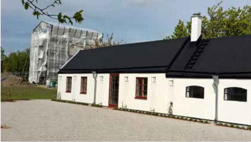
Figure 30. The Wennergren farm has been renovated while the Korsbäck Mill is still undergoing renovation in May 2016. Photograph Kopljär 2016
