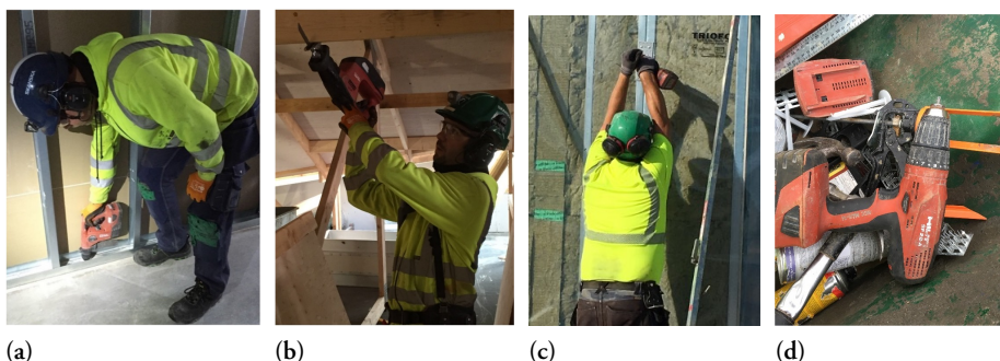
Figure 3: Carpenters using an impact drill (a), a reciprocating saw (b) and a driver (c), and tools collected in a wheel barrel to be used by a carpenter during a day (d).
