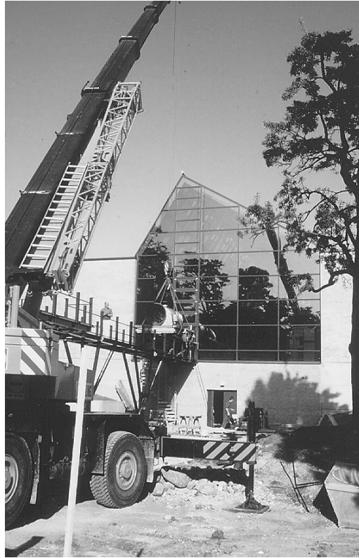
Figure 5.39 Oncological Clinic, Lund University Hospital. The picture was taken during the fan pressurisation test (Wall & Blomsterberg, 1994).
