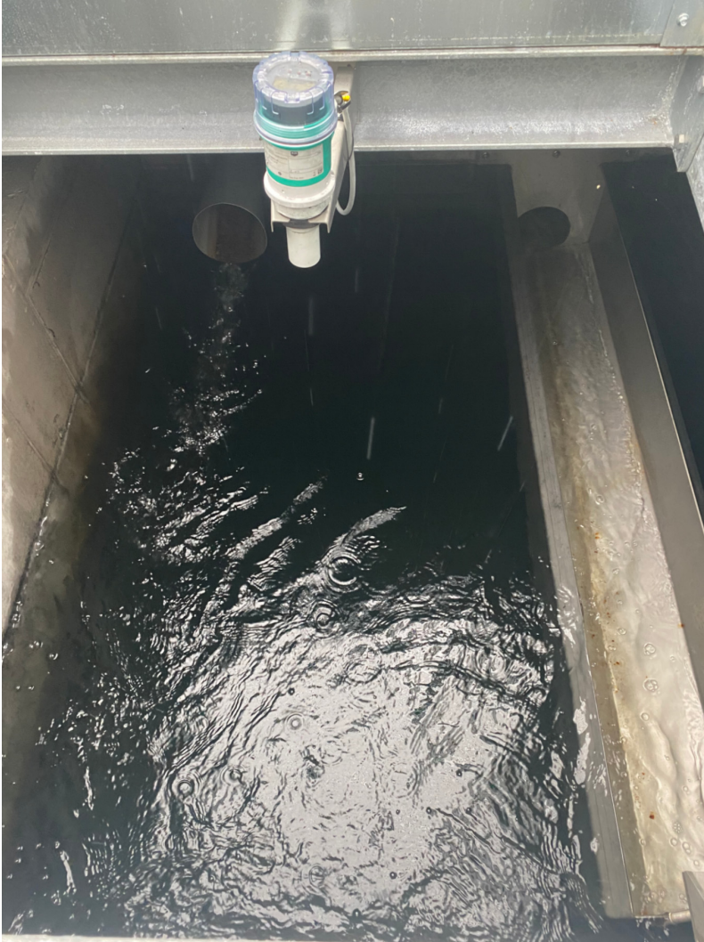
Figure 6. Photograph of GAC filter at S:t Olof WWTP. Photograph by Moa Jinbäck.
