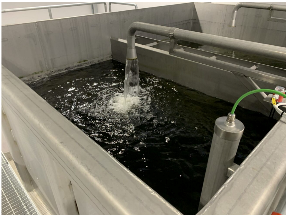
Figure 8. Photograph of GAC filters at Degeberga WWTP. Photograph by Ola Svahn.
