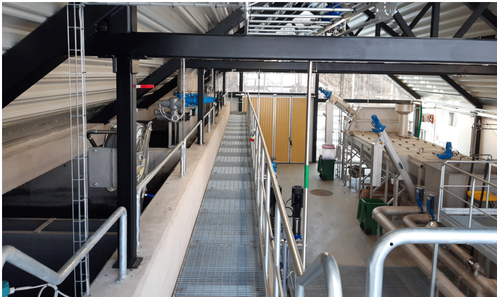
Figure 4. Photograph of parts of Kivik WWTP, with the GAC filters to the left.
