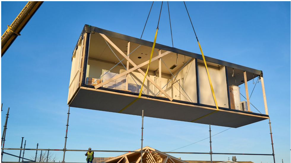
Figure 12: Timber module lifted into place. Photograph by Moelven Byggmodul used with permission.
