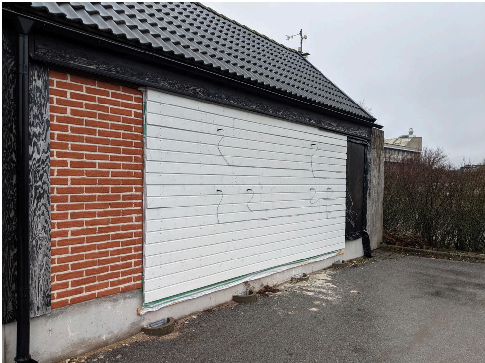
Figure 25: Southern facade with humidity sensors that are installed in the air gap between the timber cladding and weather barrier.
