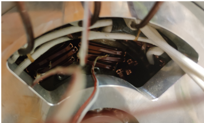
Figure 6.10: Photo of two thermocouple sensor inserted between the turns of two different coils.
