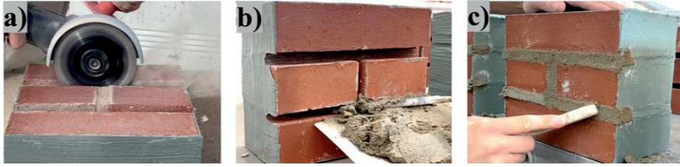
Figure 30. Different steps of repointing a specimen: a) raking out joints, b) applying new mortar, and c) compaction of the mortar [135]
