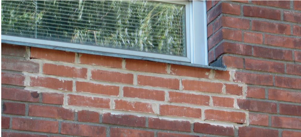
Figure 3. An example of the adverse effects of selecting unsuitable mortar and shoddy workmanship during the replacement of bricks due to frost damage
