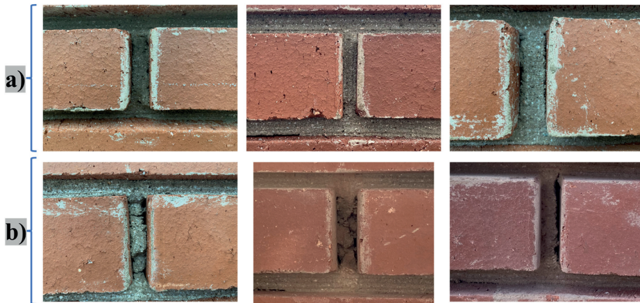
Fig. 12. Condition of head joints after being raked out to 25 mm – 30 mm: a) good/acceptable workmanship and b) poor workmanship.
