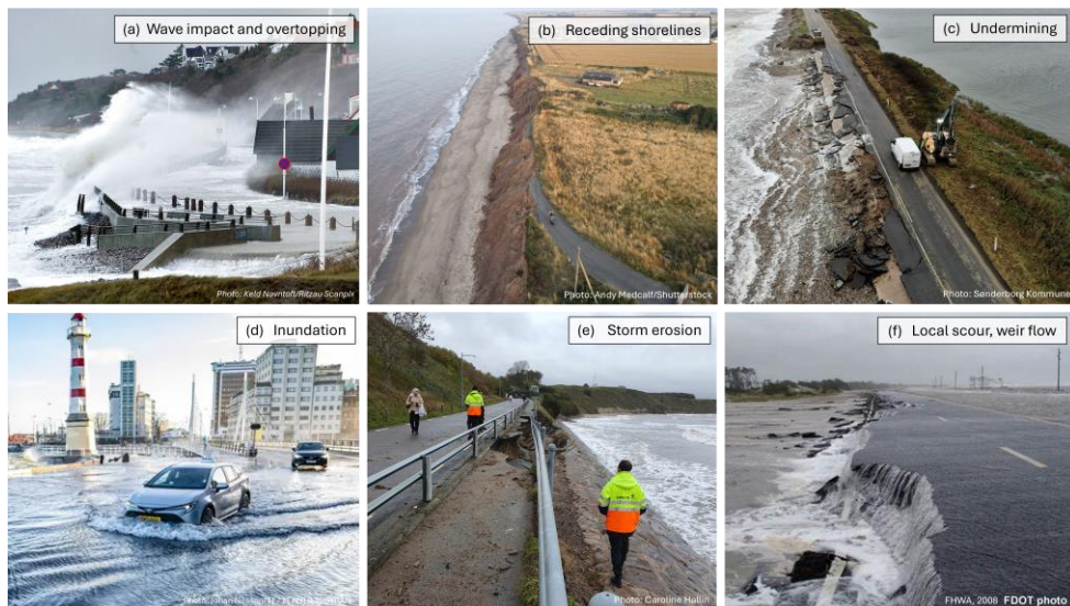
Figure 2.1: Hazards that can impact coastal roads. (a) Wave overtopping at Rågeleje, Denmark during storm Bodil in December 2013, Photo: Keld Navntoft/Ritzau Scanpix. (b) Receding shorelines, cliff erosion at Tunstall beach, UK in August 2022, Photo: Andy Medcalf/Shutterstock. (c) Road damaged due to undermining following storm erosion during storm Babet October 2023, Photo: Sønderborg Kommune. (d) Inundated intersection in Malmö, Sweden during storm Malik in January 2022, Photo: Johan Nilsson/TT Nyhetsbyrån. (e) Undermining of road at Kåseberga, Sweden, caused by wave runup during storm Babet October 2023, Photo: Caroline Hallin. (f) Local scour caused by weir flow mechanism, Photo: FHWA, 2008. FDOT photo
