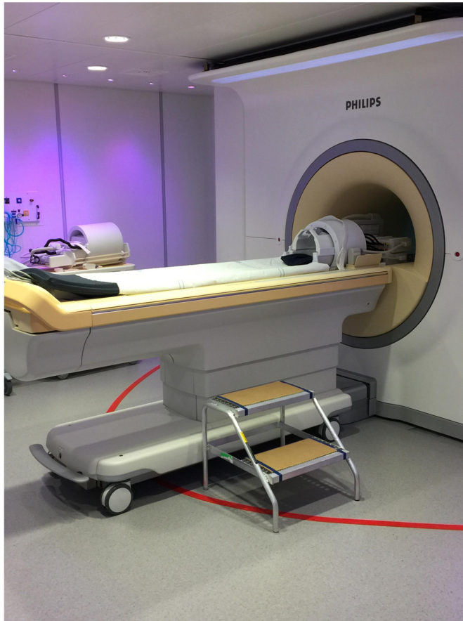
Figure 6. 7T MRI scanner installed in Lund in October 2015, by Lund University Bioimaging Center.
