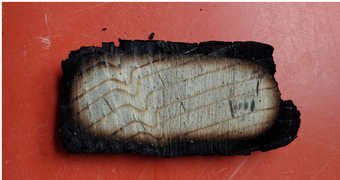
Figure C.9. A cross section of a burned timber beam showing the residual cross section which can still carry load.
