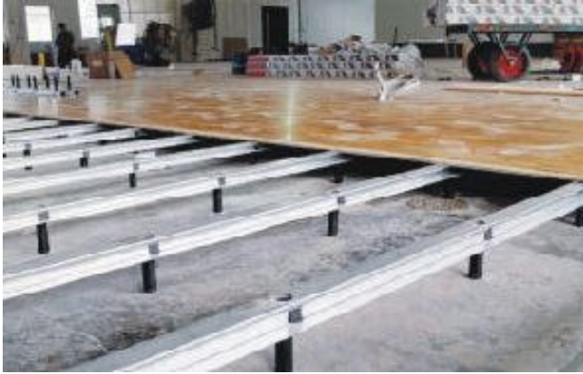
Figure 5.2 As alternative to top layer of concrete cast in-situ or self-levelling screed, some type of sub-floor system on steel girders can be used.
