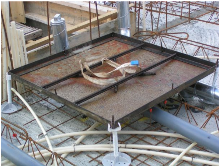
Figure 4.6 Utilisation of specially designed top formwork during casting in Case 4 led to the ability of achieving proper slopes for drainage gutters directly.
