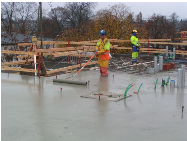
Figure 4.8 In Case 2 specially made top formwork was utilised in combination with SCC in order to achieve lower heights for slopes for drainage gutter. Note that the major part of the slab area was possible to cast with one and the same type of SCC based on increased adaptation grade to SCC compared to Case 1.
