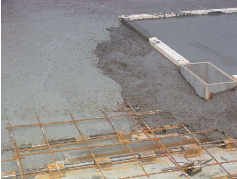
Figure 4.5 Ordinary concrete that limits the spread through the temporary wooden formwork was chosen in the wet rooms of Case 2 in order to achieve lower surface than for the rest of the slab. All other parts of the slabs were cast using SCC.
