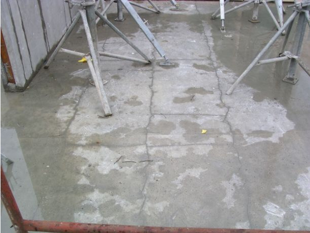
Figure 4.15 Setting cracks parallel with and above top reinforcement bars.
