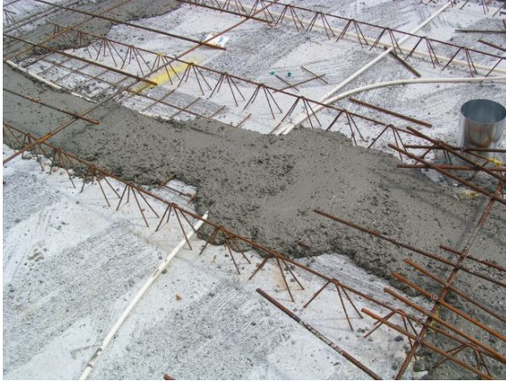
Figure 4.9 In order to avoid leach of high flowable SCC between formwork joints, the first concrete delivery for each slab casting consisted of SCC with reduced slump flow, which was placed by moving the pump mast over the interfaces.
