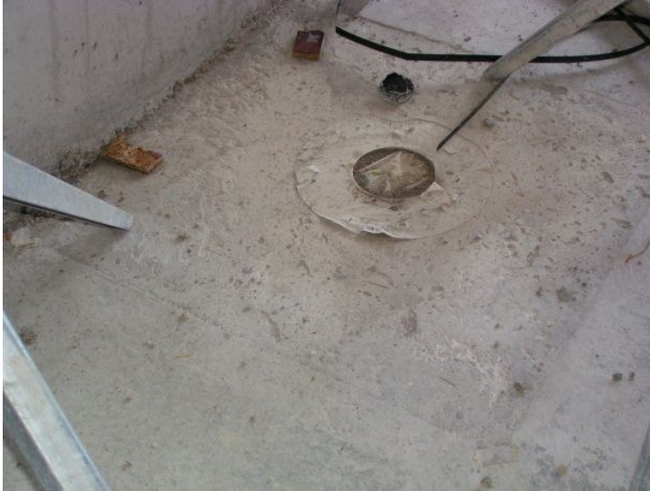
Figure 4.7 Example from Case 4 showing slope for drainage gutter in wet room directly achieved by SCC and top formwork.
