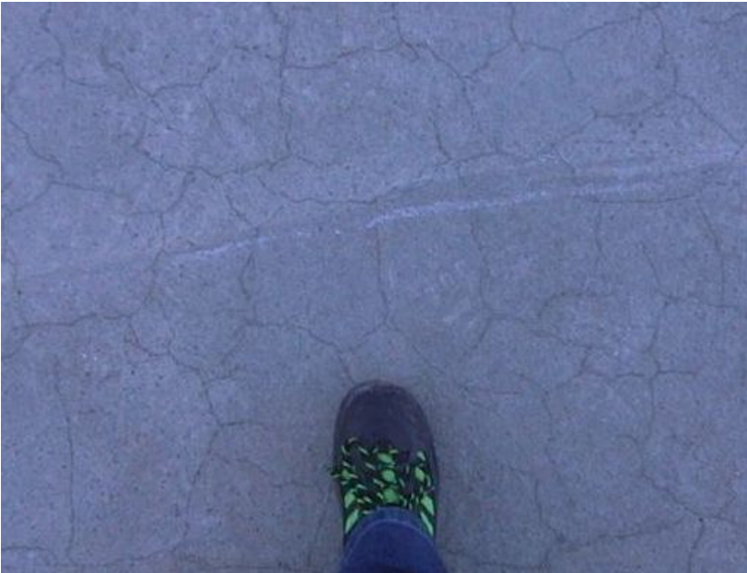
Figure 4.16 Example of heavy plastic shrinkage on slab cast with SCC.
