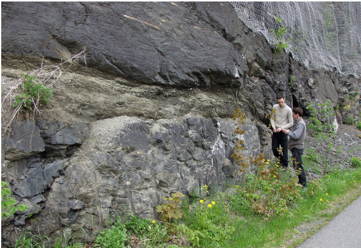
Fig. 86. A greenish, readily weathering bentonite bed (Kinnekulle K-bentonite), approximately 1 m thick, within the dark shales of the Arnestad Formation. Photo: H.A. Nakrem.
