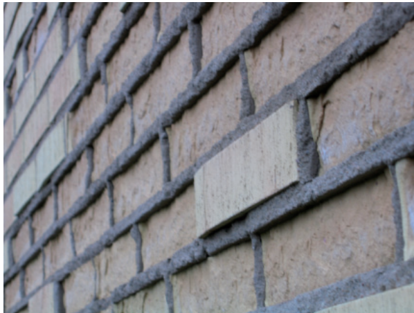
Figure 6.2 Worn out façade brick.
