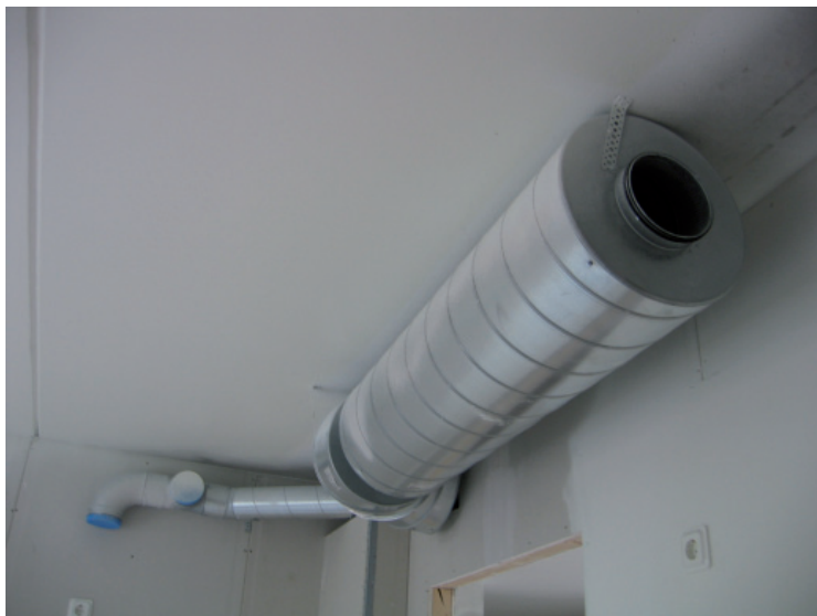
Figure 4.3 Silencers mounted in the ceiling in the apartments in Frillesås.
