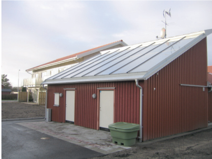
Figure 4.4 Solar collectors on the roof of the apparatus building.
