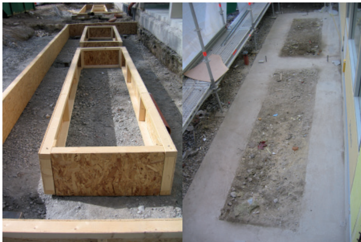
Figure 6.21 Plinths for balconies cast separate from the building construction to avoid thermal bridges.
