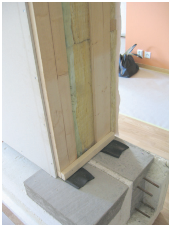
Figure 3.5 Model of wall and ground construction with the eps-insulation at bottom, the double concrete ground construction and the long side wooden wall.
