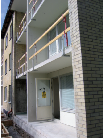
Figure 6.20 Long side walls when the outer part of the existing balconies were sawn off.
