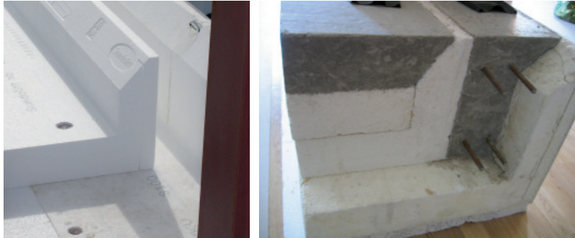
Figure 3.6 Insulation of foundation construction with the double eps foundation insulation to the left and to the right; the eps insulation filled with the load bearing concrete construction.
