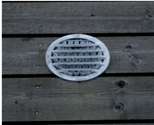
Figure 7.8 Air intake covered by rime.
