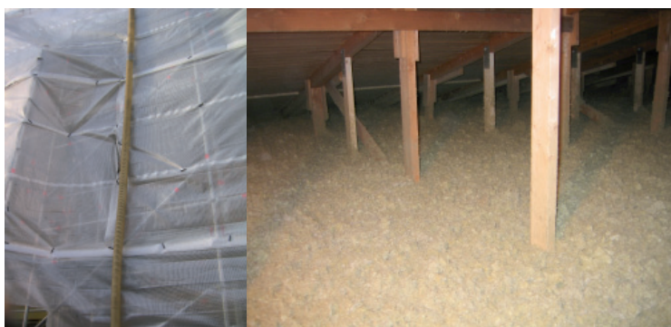
Figure 6.23 Pipe for loose wool insulation, added in the attic.
