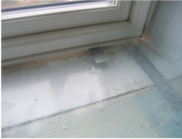
Figure 5.18 Additional metal plates in window opening to be able to mount the windows.
