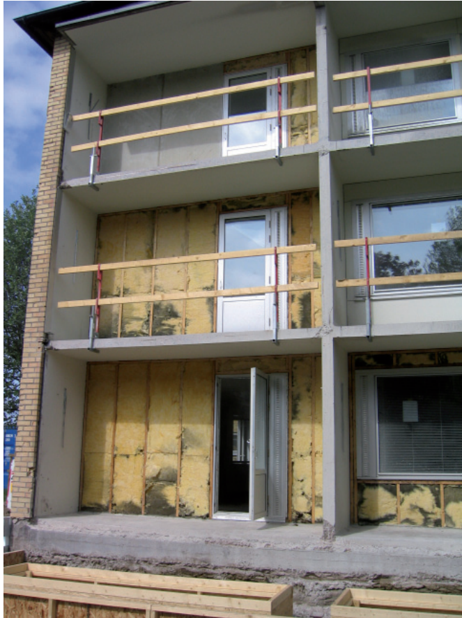
Figure 6.16 Discoloured mineral wool insulation.
