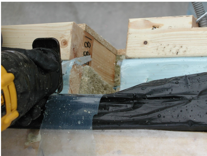
Figure 7.22.2. Location of the studied position before the sensor, the iron beam, the slab and the wall on the second floor was mounted.
