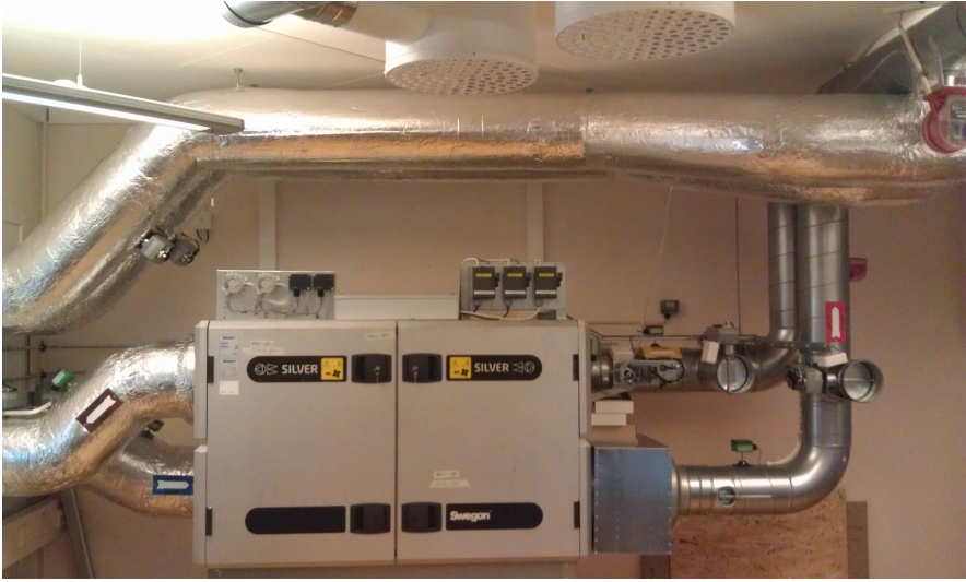
Figure 26. The air handling unit.
