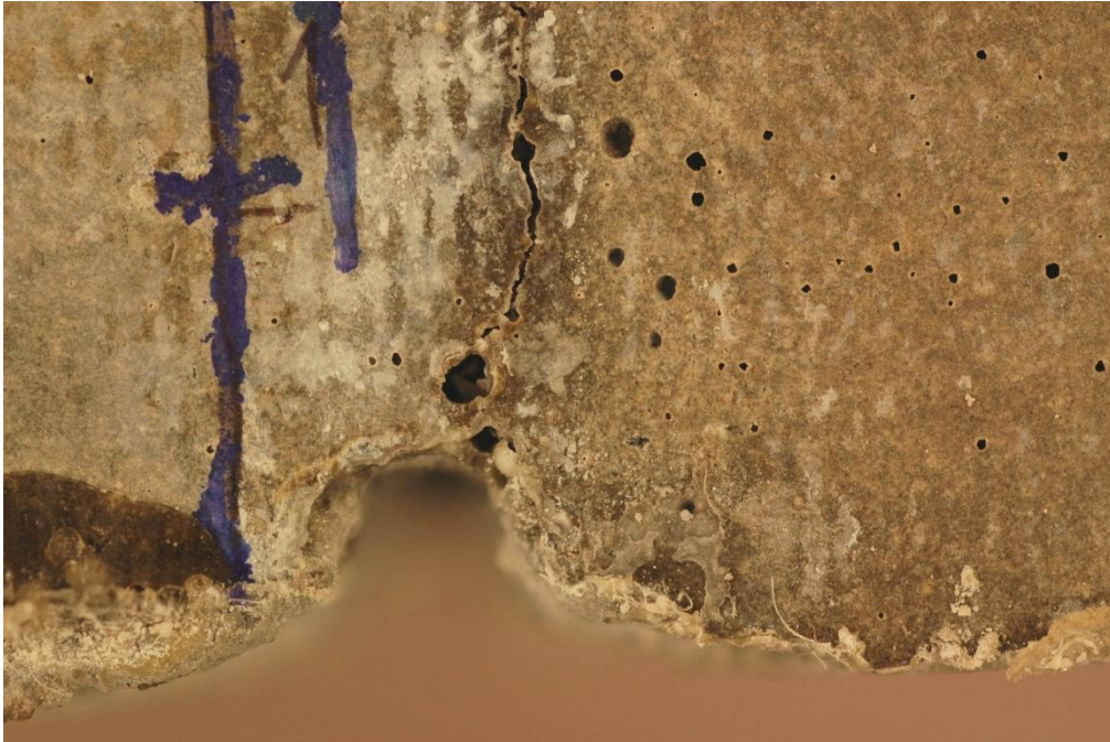
Figure 12.2: 0.2 mm crack after 1 year permanent immersion in sea water. Test series 1, specimen H75-2-1-1.
