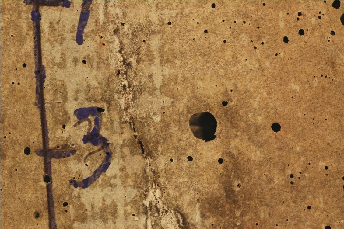
Figure A2.1: 0.2 mm crack after 1 year permanent immersion in sea water. Test series 1, specimen H75-2-1-1.
