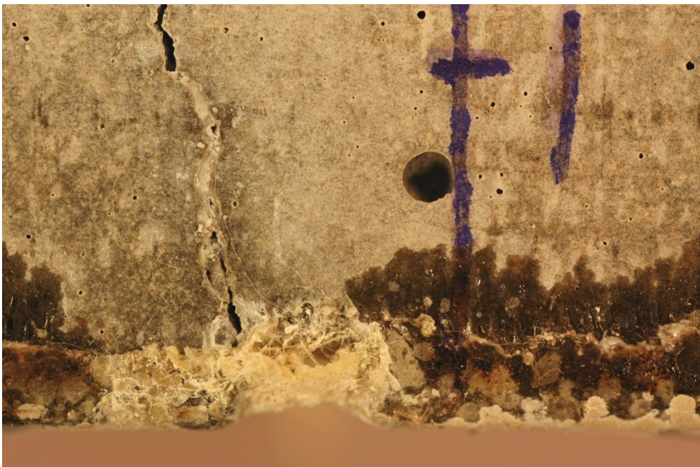
Figure 12.3: 0.4 mm crack after 1 year permanent immersion in sea water. Test series 1, specimen H75-4-1-1.
